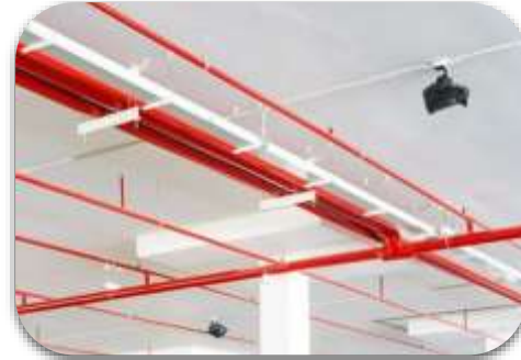
FIRE SPRINKLER SYSTEM
