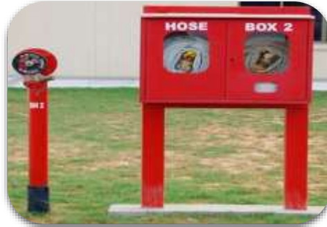
FIRE HYDRANT SYSTEM
