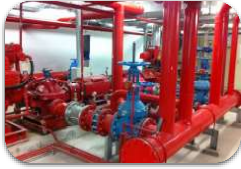
FIRE UNDERGROUND PUMP ROOM
