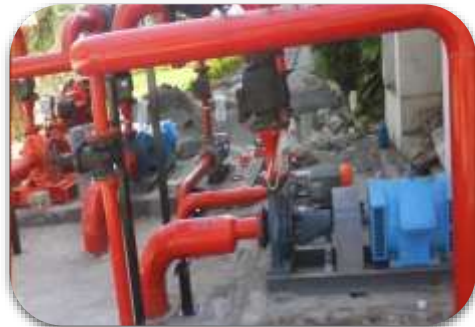
FIRE ABOVE GROUND PUMP ROOM
