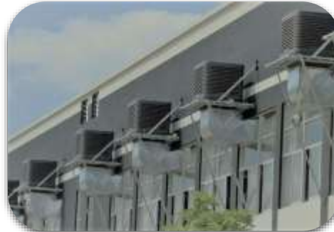
CENTRAL AIR COOLING SYSTEM
