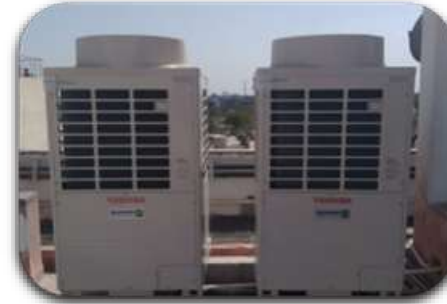
VARIABLE REFRIGERANT FLOW (VRF/VRV)
